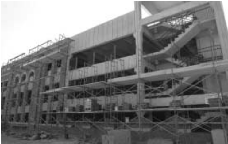
Progress is moving so fast that any picture of the new parking garage on Fourth Avenue South will be out of date as soon as it's taken. The facade is now nearing completion.
